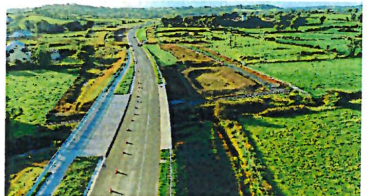
Aerial view south of the new N55 Mainline in the vicinity of Bridge 1 in the townland of Killydoon.
