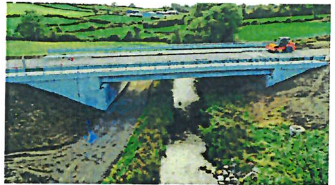
Aerial view of the progress at Bridge 3 in the townlands of Ballytrust Lower and Legwee.
