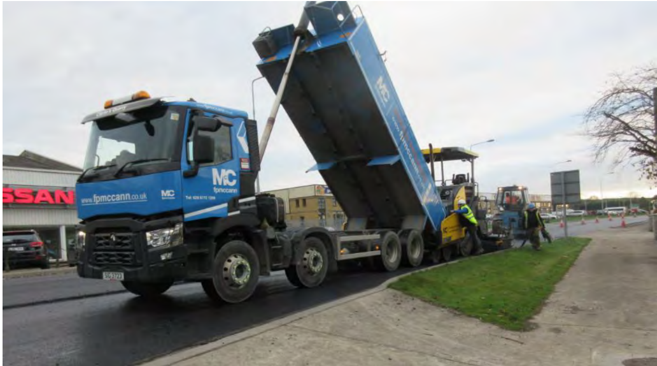
Photo showing surfacing works on the N55 Moynehall to North Ballinagh Pavement Overlay Scheme
