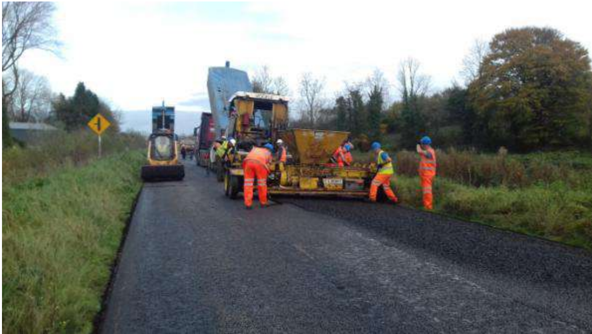
Photo showing Chip laying crew on the N87 Lisnamaine to Rahaghan Pavement Overlay Scheme
