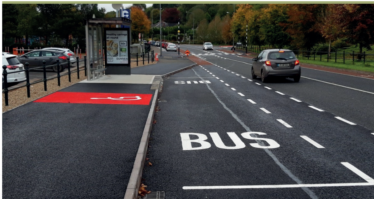
Fig 7.1 New bus bays, cycle path & pedestrian crossing at Cavan Institute of Technology 2019
