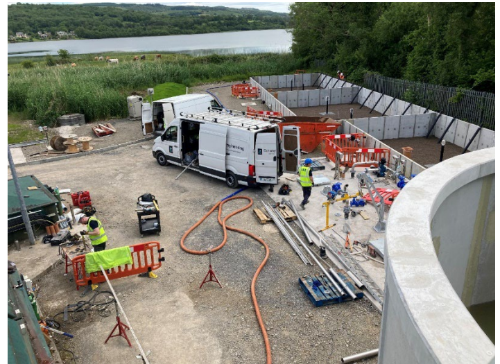
Sludge Drying Reed Beds and Mechanical Fit out
