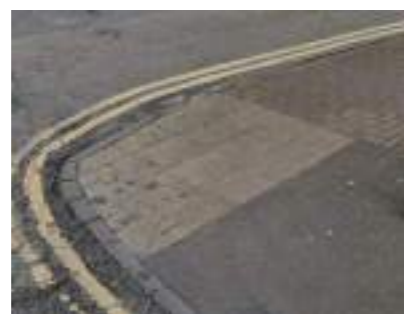
Figure 91 - Pavement at Thomas Street
