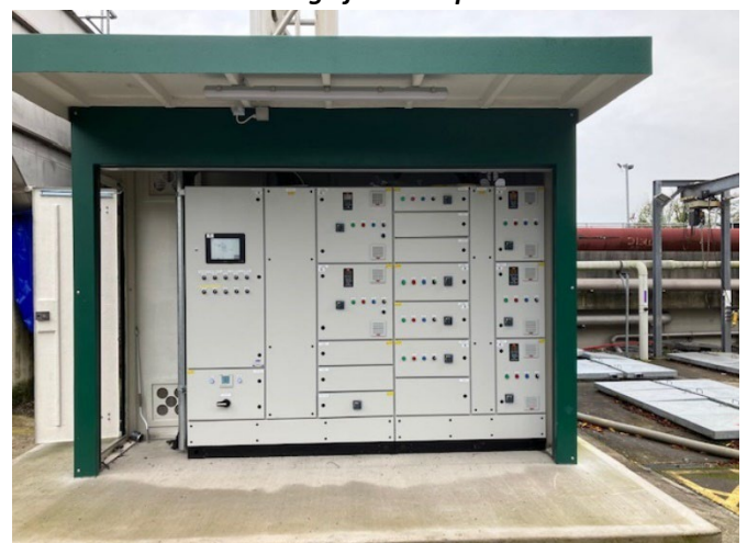
New Panel & Enclosure
