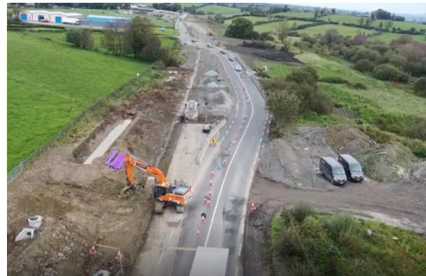
Above: Aerial view of the temporary diversion constructed near the southern tie-in to facilitate construction of the Mainline.
