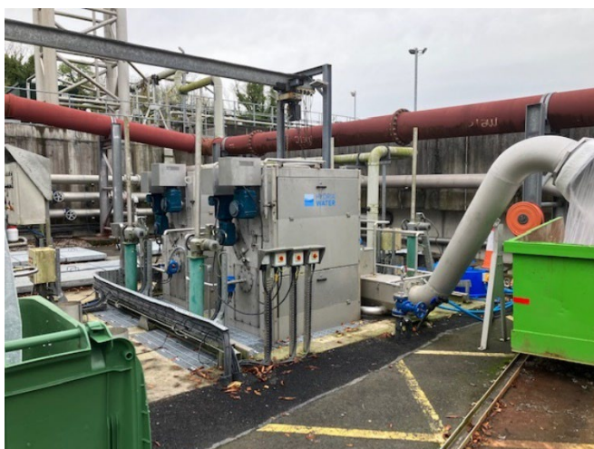
Two New Screens and Handling Unit
