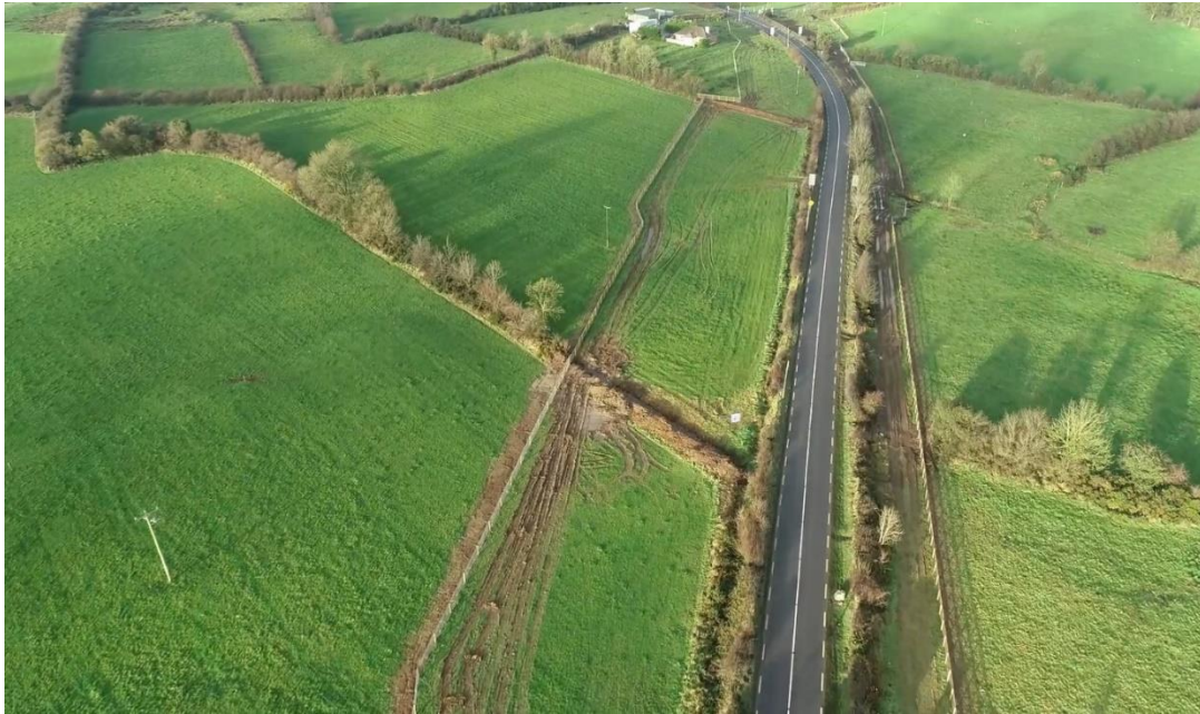
Above: Aerial view of boundary fencing works on the N55 Corduff to South of Killydoon
