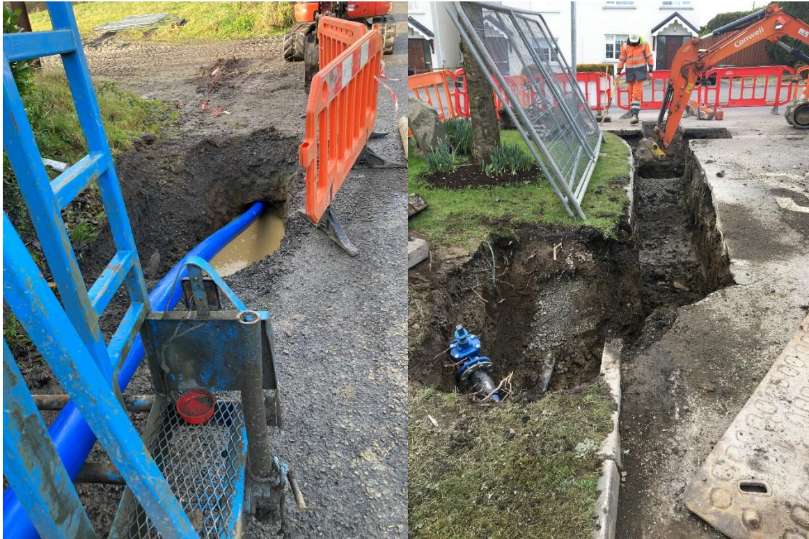
125mm HDPE pipe installation by directional drilling at Shankill Billis (left) and works on Back Yard Services in Belturbet (right).
